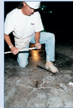
The existing concrete and terrazzo floors in the 18,500-sq.-ft. retail location space were cracked and uneven.
