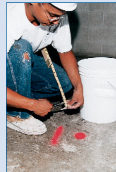
Based on the laser results, elevation pins were attached to the floor to indicate how thick the underlayment should be applied.
