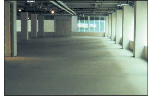
The new gypsum concrete underlayment provides a smooth, even surface, ready for floor finish material installation. The entire application was completed for less than half the cost of using a portland cement-based product.
