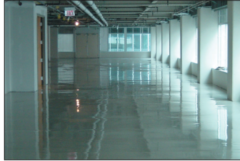
Approximately 525,000 sq. ft. of gypsum concrete underlayment (shown freshly poured) was applied over the existing floors throughout the building.
