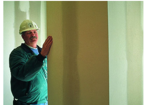
Drywall corners treated with paper faced bead “float” with the gypsum board surface, providing the flexibility needed to withstand structural shifting and wood frame shrinkage without cracking.
